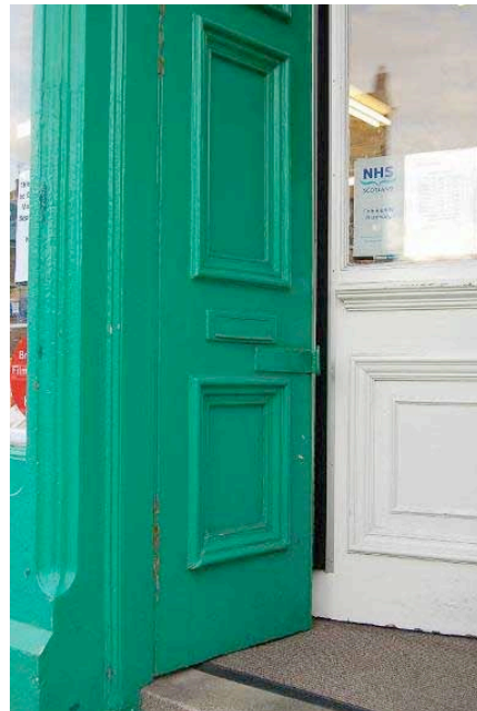
Shop storm doors
