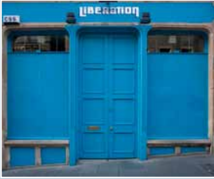
Cockburn Street, Edinburgh. Original later 19th-century timber panelled security shutters that slide down into slots beneath the windows during the day. © N Haynes.
