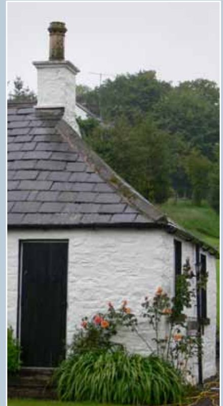
Regular courses, but random widths of local slate fixed using a double-lap method under stone ridge pieces. Dumfries & Galloway.
