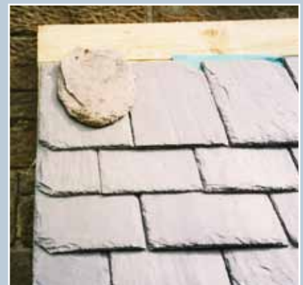
Sample panel prepared to ensure appropriate grading and random widths in the laying of new slate, with a fire-damaged Perthshire slate from Morgan Academy, Dundee.
