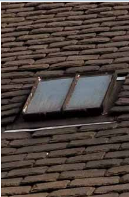
A traditional iron rooflight set into a West Highland slate roof. The small size, low profile and 'portrait' format are typical characteristics. © N Haynes.
