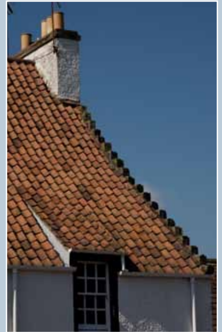
Clay pantiles and a 'catslide' dormer on a 17th-century house, Falkland, Fife. The roof sweeps up a little towards the eaves. © N Haynes.
