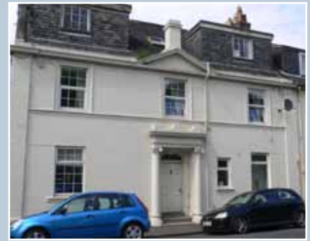
Badly designed box dormers detract from the classical proportions and elegant detailing of this late 18th-century house.
