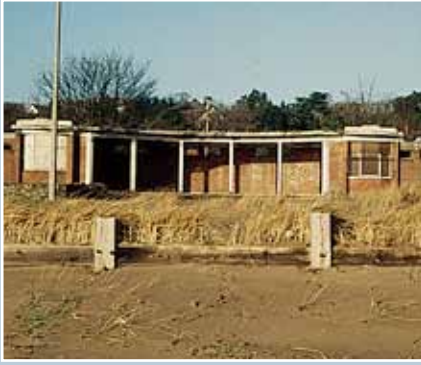
C(S)-listed Art Deco beach shelter at Broughty Ferry, City of Dundee. Consent was refused for demolition because the building was not marketed adequately.
