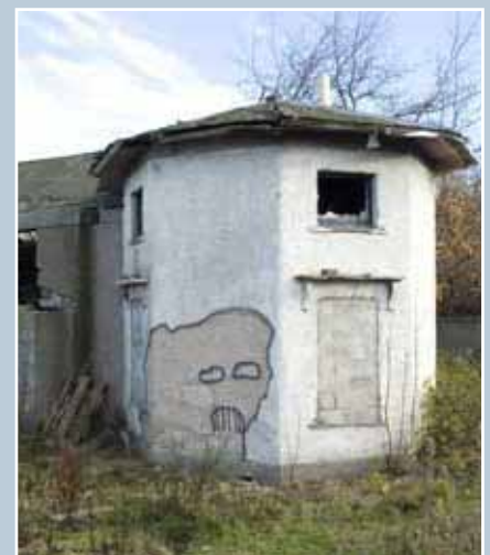
A category B-listed toll-house of circa 1830 at Great Northern Road, Aberdeen. Consent was granted for demolition in 2006 on the grounds of its poor structural condition, road-blighted location, and the lack of a restoring purchaser. © Crown copyright: RCAHMS. Licensor www.rcahms.gov.uk .
