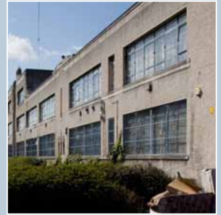
Former Niddrie Marischal School, Edinburgh. Designed in Art Deco style in 1935 by architects Reid & Forbes. The strips of blue-painted steel windows have two opening methods: horizontal pivots and small hoppers. The ground-floor windows are protected from vandalism by discreet metal mesh screens painted in the same colour. © N Haynes.
