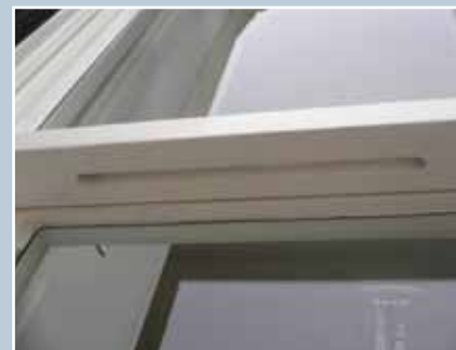
A view of the underside of the meeting rail of a new timber sash and case window at Castlemilk Stables, Glasgow. A discreet slot ventilator in the meeting rail allows ventilation without the need for obtrusive external fixtures.
