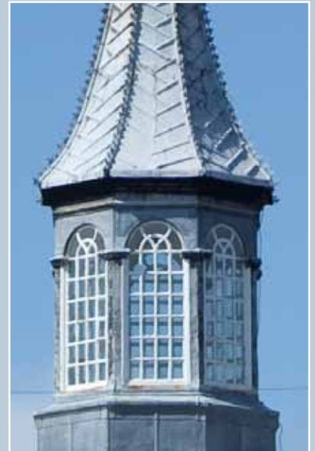
Fixed small-pane windows in the cupola of Robert Gordon's Hospital, Aberdeen, designed by William Adam in 1731–32. Thick astragals (glazing bars) and small panes of glass are typical of this period of design. © N Haynes.
