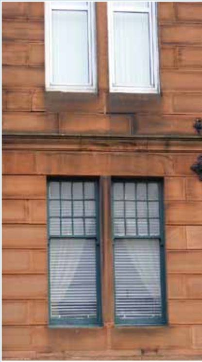
Original timber sash windows of circa 1900 at the lower floor and poor replacement windows at the upper floor. The historic character of small-pane upper sashes and dark-painted frames is lost through use of modern plastic materials, a non-traditional opening method and clumsy profiles designed for double-gazing.
