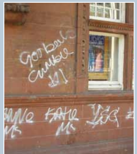
Graffiti: The removal of graffiti requires prompt action before the paint or ink dries into the wall surface. Cleaning methods should be tested on a small unobtrusive area to determine the least aggressive treatment for effective removal of the graffiti. In extreme cases of repeated vandalism, a sacrificial wax coating might be considered for vulnerable surfaces.
