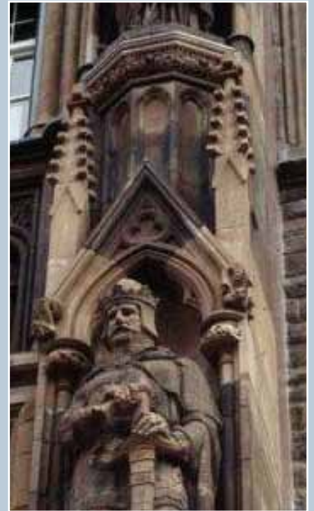
Scottish National Portrait Gallery, City of Edinburgh, 1890. Decisions about whether to re-carve stonework are a matter of values. Here the artistic value of a sculpture calls for it to be conserved mostly as found, whereas the architectural elements (finials and hoodmoulds) that also function in shedding rainwater have been completely replaced where required. © Copyright: RCAHMS (William McKelvie Collection). Licensor www.rcahms.gov.uk .
