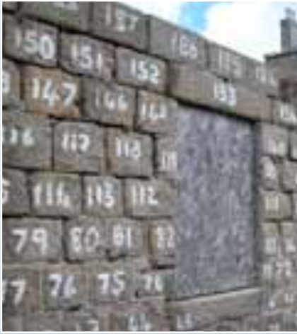
Structural instability requires the rebuilding of this wall in Peterhead. The granite stones have been numbered ready for reinstatement.
