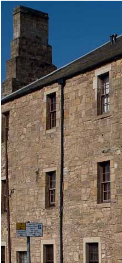
The exposed wall of this 17th-century house in Cupar, Fife, reveals archaeological evidence of a number of blocked openings. The previous mixture of window sizes and levels has been regularised in the current arrangement. © N Haynes.
