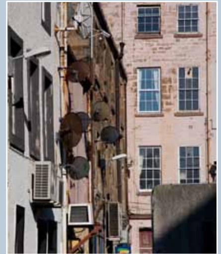
The cumulative effect of modern fixtures, including satellite dishes, air conditioning units, signage and street lighting, is damaging to the character of this 18th-century building.
