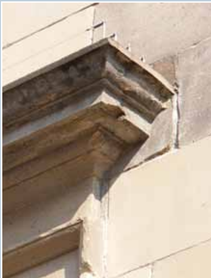
Discreet sprung wires are attached to the top surface of this cornice to deter birds. Miller Street, Glasgow.
