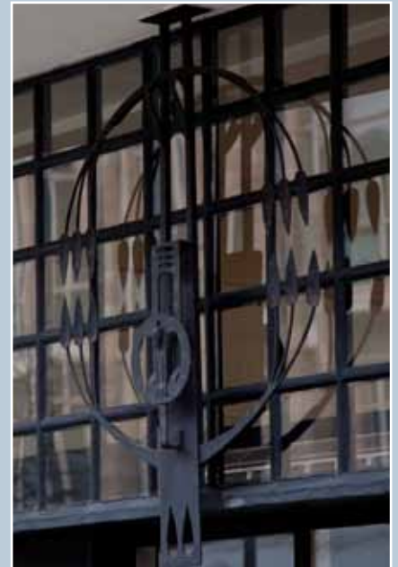
Decorative ironwork by Charles Rennie Mackintosh fixed to the exterior of the Willow Tea Rooms in Sauchiehall Street, Glasgow. © N Haynes.
