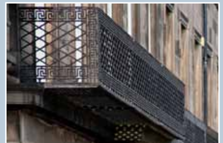
A cast-iron balcony marking the principal room on the first floor of a townhouse in Regent Terrace, Edinburgh, part of the development planned by William Henry Playfair in 1825 and built 1826–33. © N Haynes.
