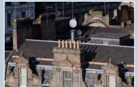
These satellite dishes are positioned in a roof valley and are not visible from street level. Fixed to later service features they do not damage architectural details. © N Haynes.
