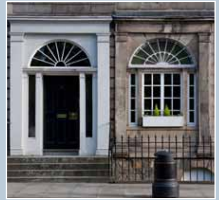
The old conversion of the right-hand doorway to a window and removal of the main entrance steps is disruptive to the character of the building and the broader pattern of entrances and windows in the street. © N Haynes.
