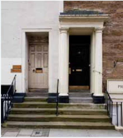
Removal of the left-hand doorcase has unbalanced this pair of entrances. © N Haynes.
