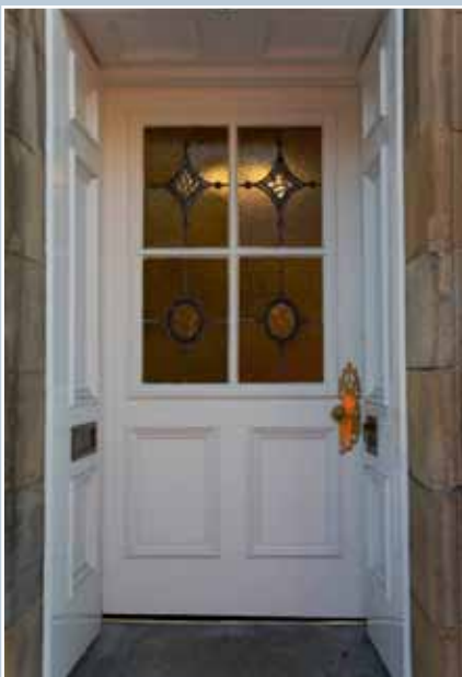
A late 19th-century two-leaf outer door and an inner vestibule door with decorative leaded glass panels in Falkirk. Associated fixtures include the brass letterbox and door handle to the outer door and the brass doorknob and decorative finger-plate to the inner door. © N Haynes.
