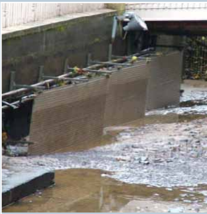
New Lanark mill lade. Receptor panels during installation for two 44kW water-source heat pumps. After installation the lade levels were returned to normal - the panels are not normally visible. © New Lanark Trust.
