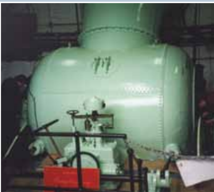
The refurbished Boving turbine (1930) at New Lanark World Heritage Site has 500 kW generating capacity. © New Lanark Trust.
