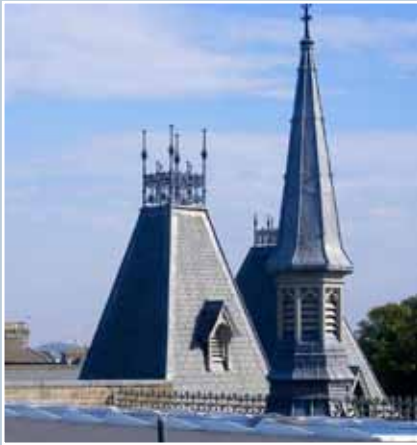
Photovoltaic panels located discreetly on hidden parts of the roof at Morgan Academy, Dundee. The panels power a ground-source heat system.
