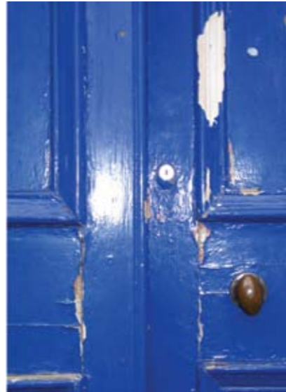
If not regularly maintained paint will begin to peel from doors leaving them vulnerable to further deterioration.
