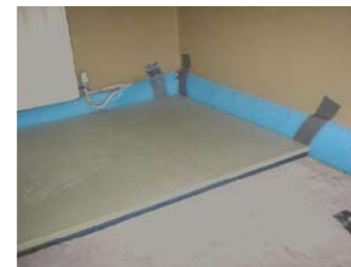
Fig 5. Addition of floor insulation to a modern concrete floor. Lister Housing Co-operative.
