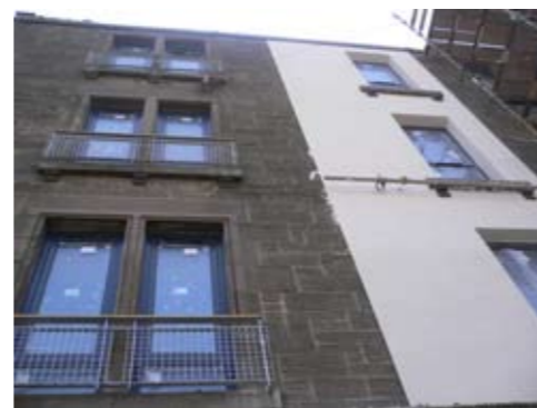
Fig 11. External insulation applied to an unlisted tenement has dramatically changed its architectural character.
