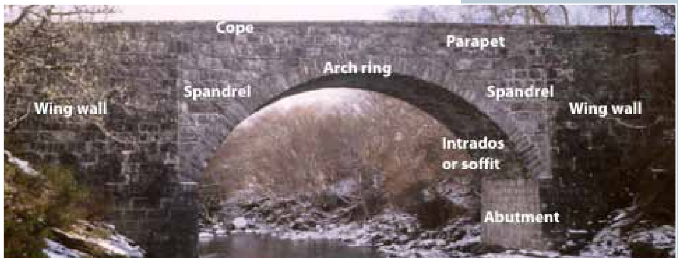
Below: parts of a bridge, identified on the repaired road bridge at Orrin, Highland.
