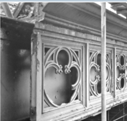
Dalmarnock Bridge, Glasgow, is a series of wrought iron girders behind a gothic cast-iron spandrel. It was strengthened in 1996 by insertion of new steelwork. The repaired cast-iron parapet is protected from traffic by bollards.
