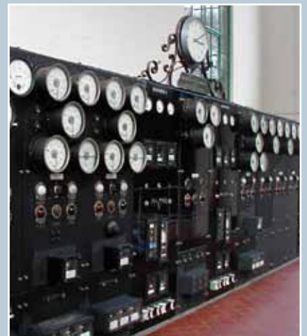
The control panel at Bonnington Power Station, South Lanarkshire, 1927, was retained in situ by Scottish Power although superseded by a computer.
