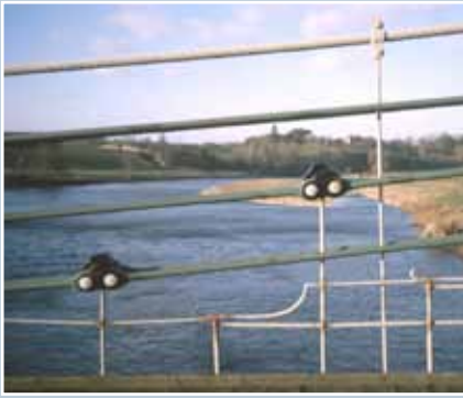
Union Bridge, Scottish Borders, 1821, the oldest suspension bridge still carrying a road, showing a clear distinction between the historic chain links and a 1920s wire cable. The deck is wooden and the parapets do not conform to modern standards. A weight limit and bollards exclude heavy vehicles.
